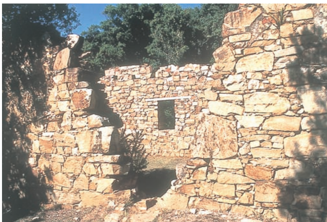
The ruins of a timber shed built under supervision of Johann Friedrich Meeding at Plettenberg Bay more than two centuries ago. It is a declared national monument
